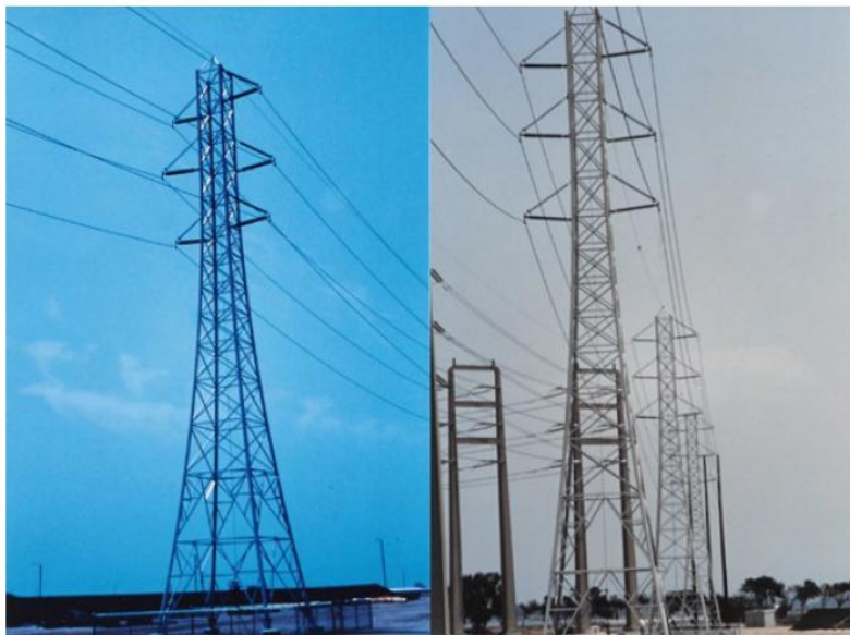
Figure 9-2 The 230 kV FRP lattice structures with composite insulators
