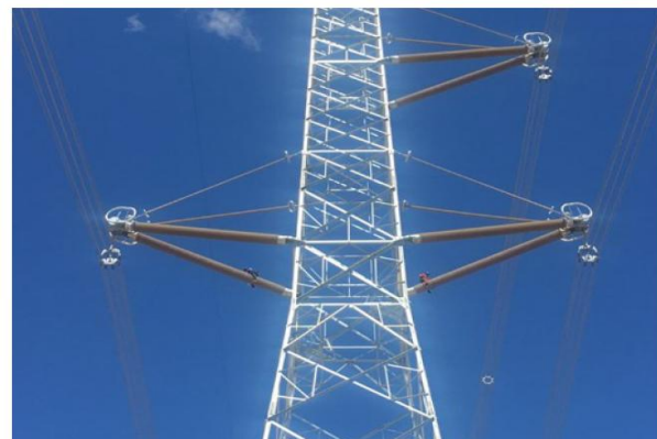
Figure 9-12 1100kV hybrid tower, steel and FRP composite.
